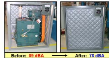
Sound dampening blankets installed around Stokes vacuum pump at the Turbine Module Center have reduced the noise level by over 10 decibels.
